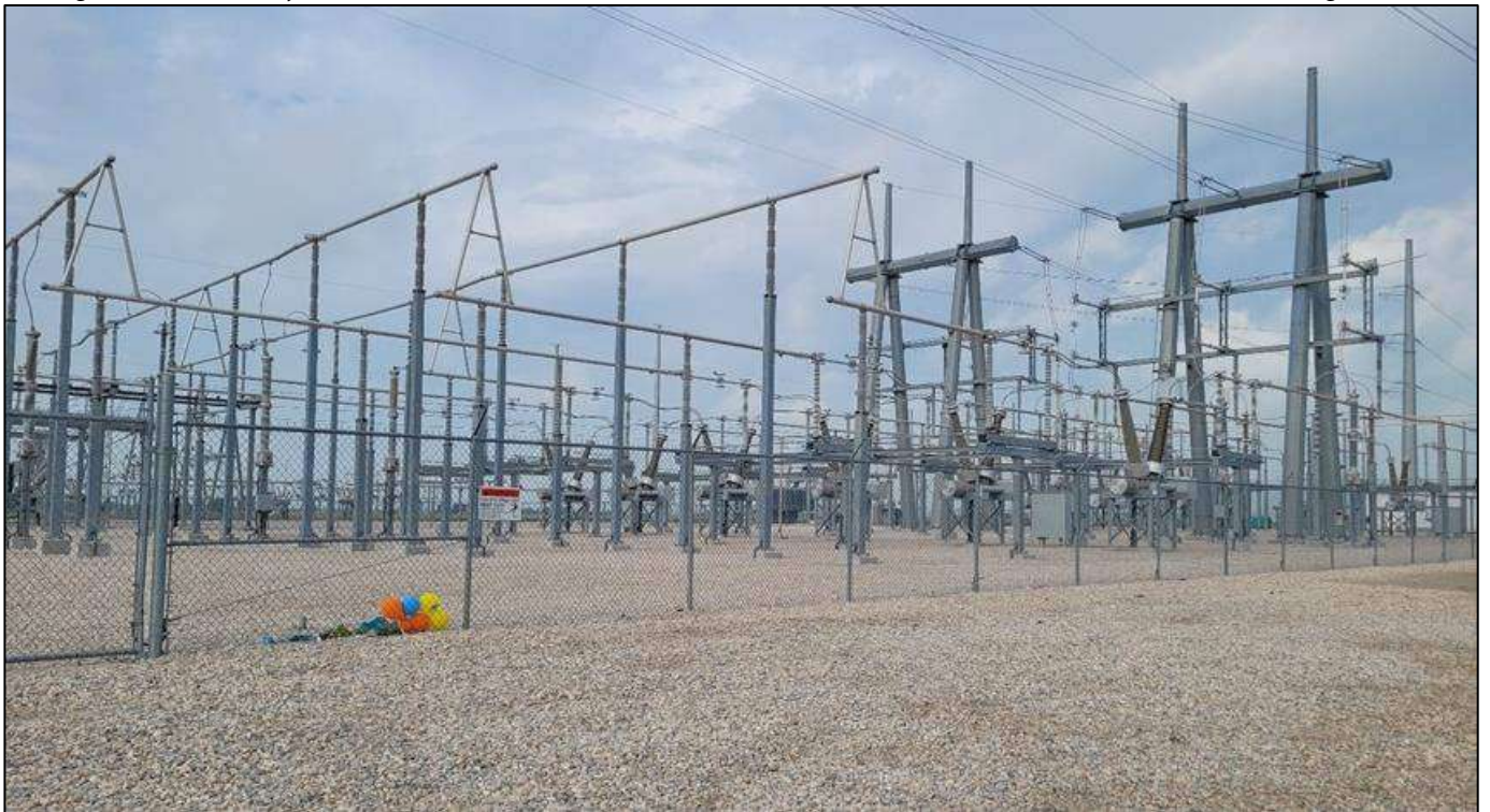
Figure 18: Indicative BESS substation image (Source: ACCIONA Energía)
