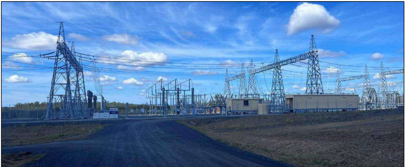
Figure 11: Development area photographs showing the adjoining Powerlink MISS (Source: Saunders Havill Group).
